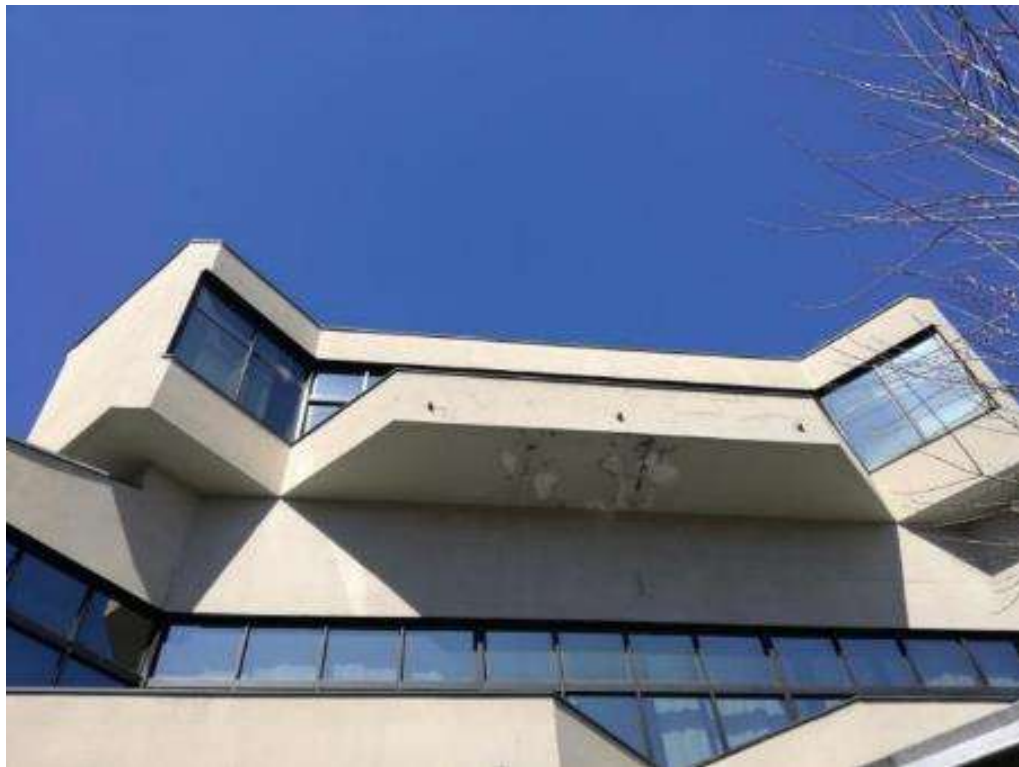
Figure 5-5 Water damage on the intrados of a terrace at the GAM
