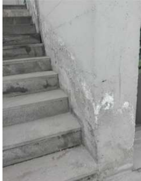
Figure 5-10 Detachment of concrete and shifting of the stair treads
