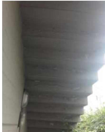
Figure 5-8 Flaking of the paint protecting the concrete
