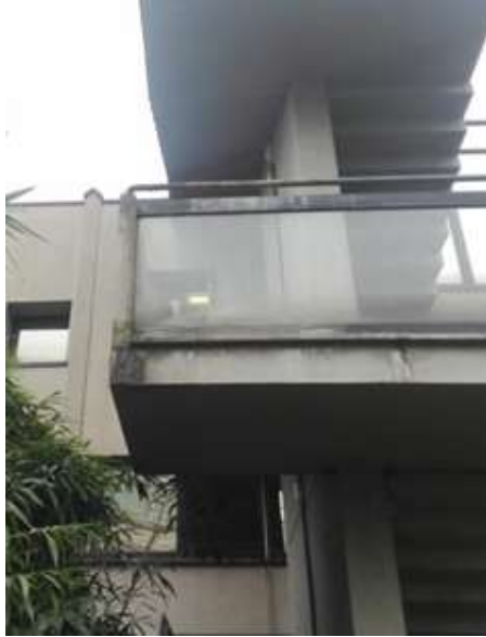
Figure 5-9 Deterioration of the landings and glass parapets
